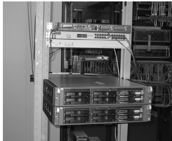
Figure 3: System Hardware at the DeLeon Central Office
